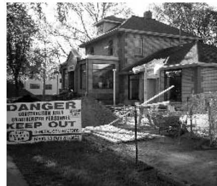
Here is a photo of the construction area surrounding the Credit Union.
