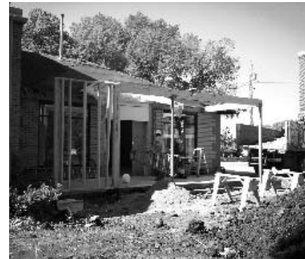
Here is a photo showing the renovation to the exterior of the Credit Union.
